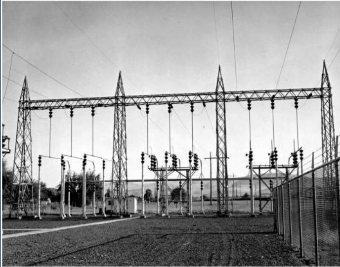
Ellensburg Substation, BPA (1951)
